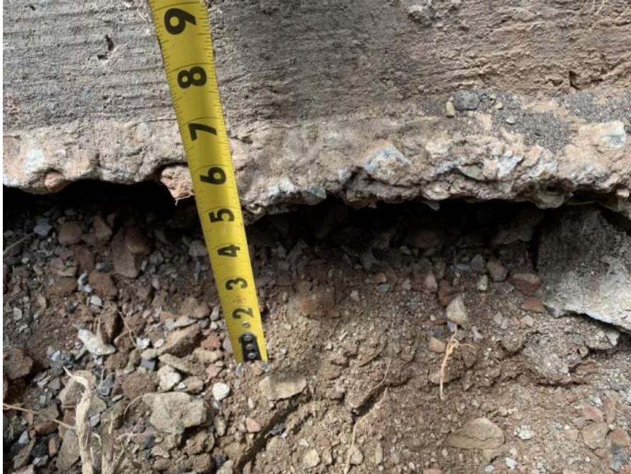
LTP-1: Existing void beneath concrete grade beam (facing west)
