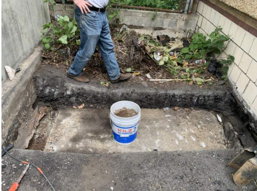
LTP-1: Adjacent to the eastern edge of the Cherry Street Bridge Abutment (facing north)
